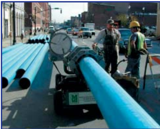
HDPE pipe for water main rehabilitation in Louisville, Ky., is heat-fused on location using equipment from McElroy Manufacturing Inc. ISCO Industries.
